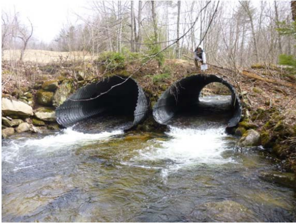
Before – perched & undersized culvert pipes
