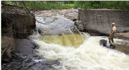
The Franconia Paper Mill dam on the Wells River in Groton, VT has blocked the river for more than 100 years.
